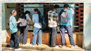
Newly Installed Water Coolers
